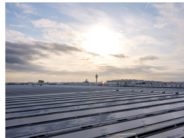
The electricity purchased by Schiphol Group comes mainly from wind, though the amount of solar is increasing.
